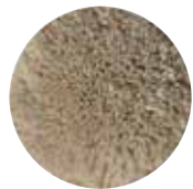
PWO1157 CT77952 Castle Wall
